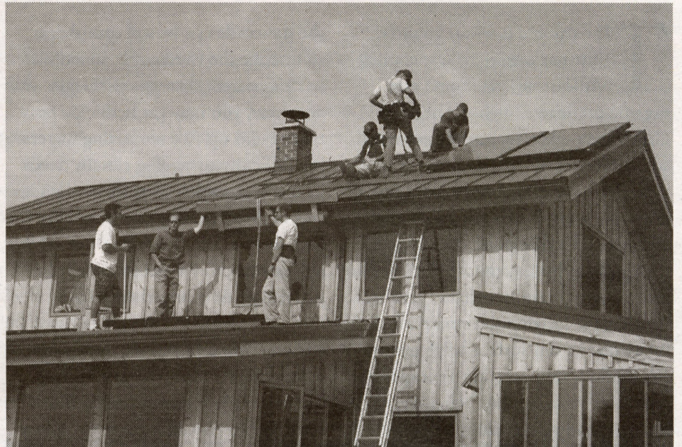
Installing the solar hot water panels on the Forbes' roof this past September.
