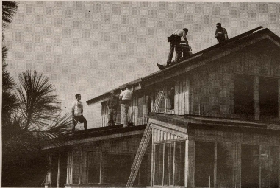
Installing the drainback solar hot water system on the roof of the Forbes family home.
