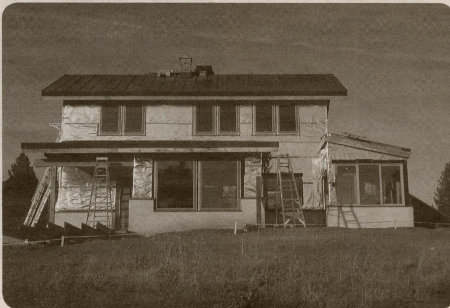
Our house wrapped in a radiant barrier.
